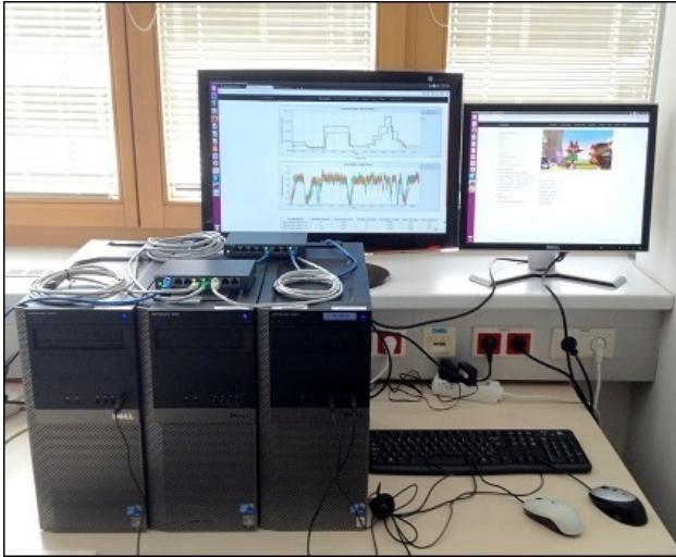
Figure 2: Picture of the Server Infrastructure.
